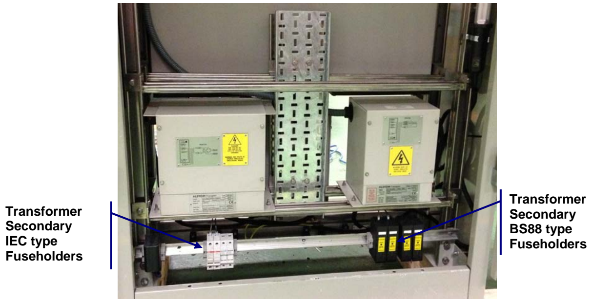
Figure 16: Transformer Secondary Outgoing Fuseholders
