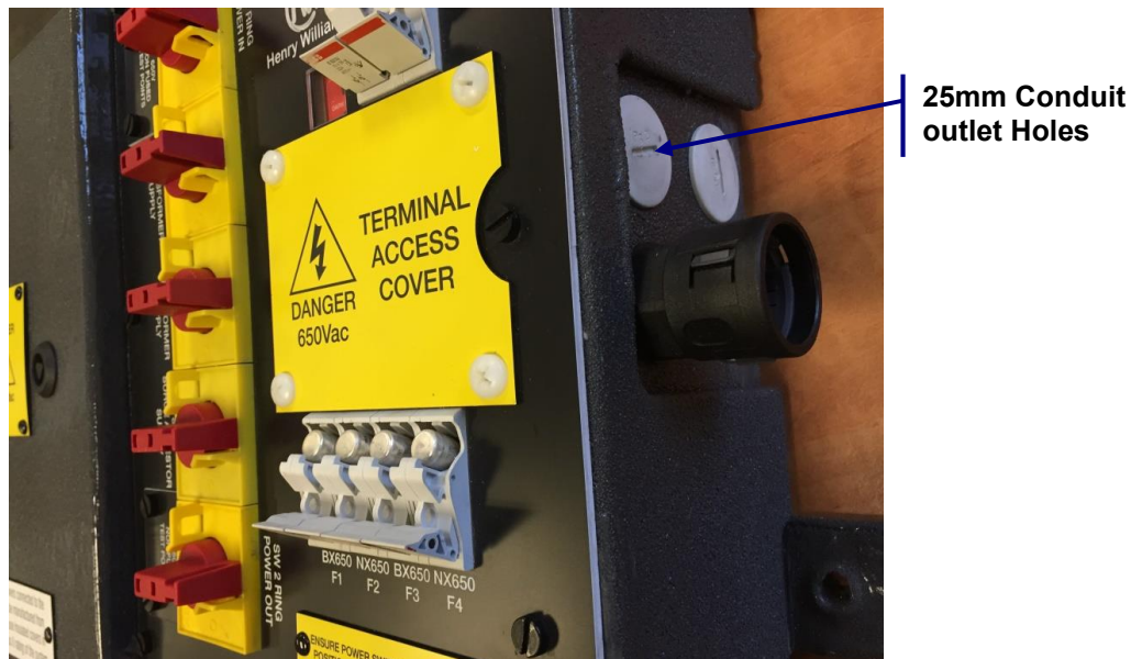
Figure 3: Functional Circuits/Transformer Wiring Outlets
