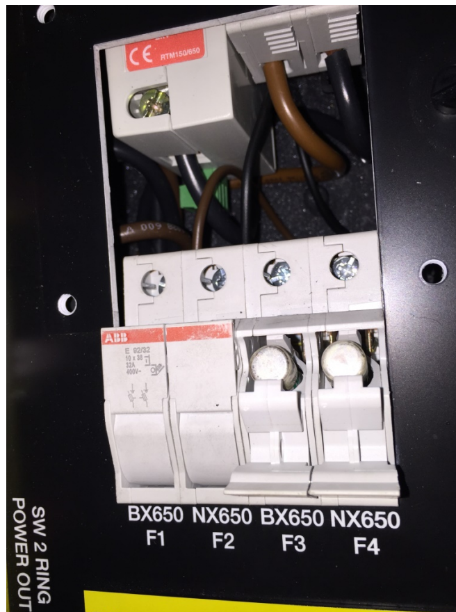
Figure 15: Functional Wiring Terminated
