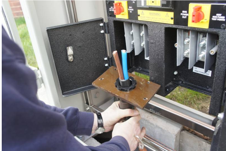
Figure 5: Cable Gland Plate removed from the enclosure
