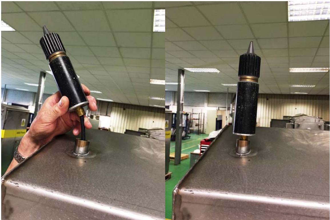
Figure 8: Installation of Precipitation Sensor
