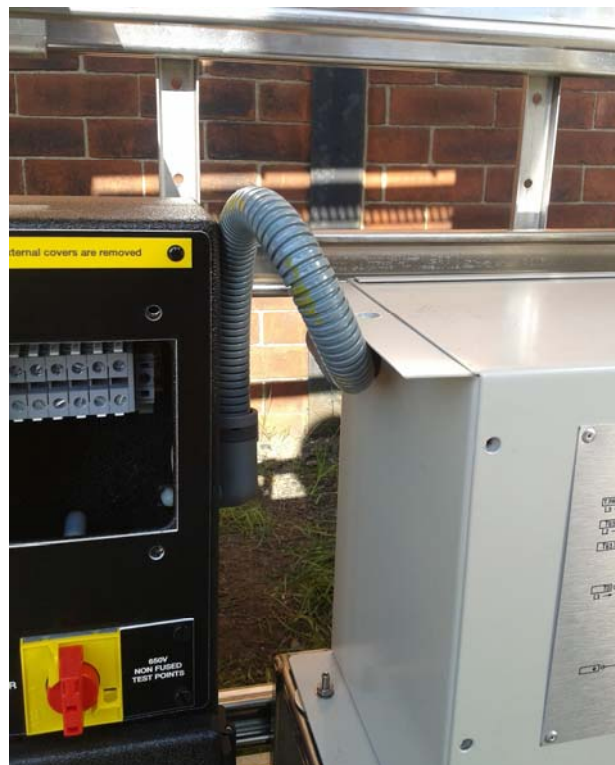
Figure 14: Termination of Hybrid Transformer Primary Feed Cables
